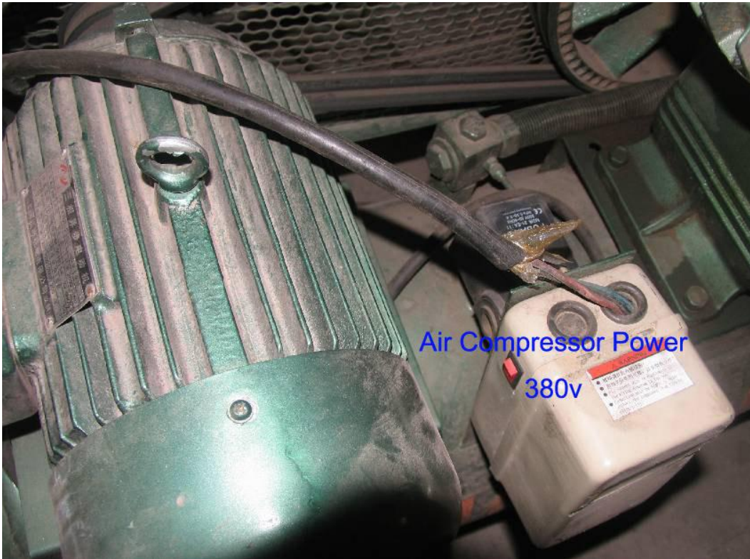
Photo 4—Air compressor power connect
