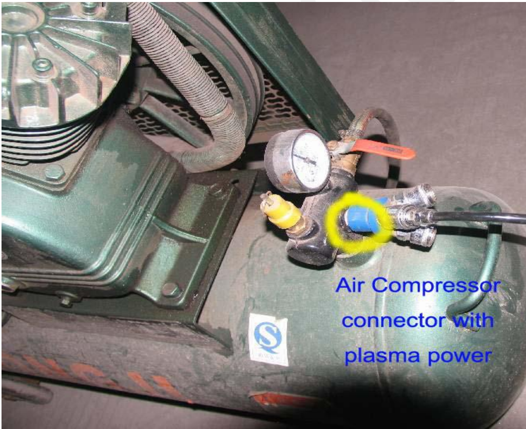
Photo 5-Air compressor connector with plasma power
