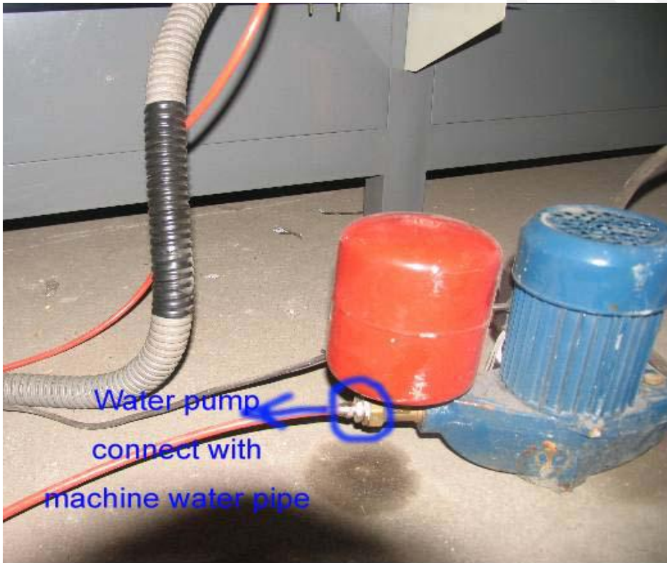
Photo 7- Water Pump connect with machine pipe
